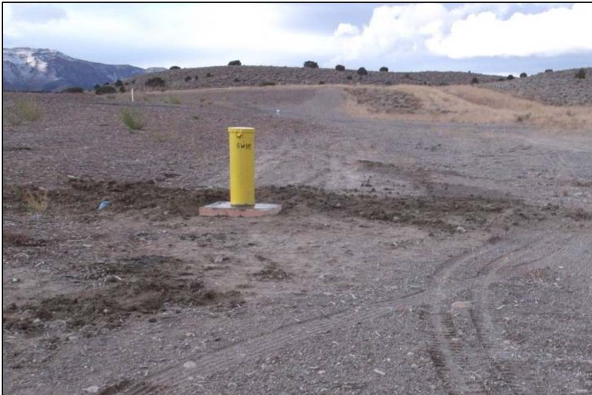
Plate 3-2. Landfill gas monitoring well GW-3R with GW-3 in background just to right (view north).
