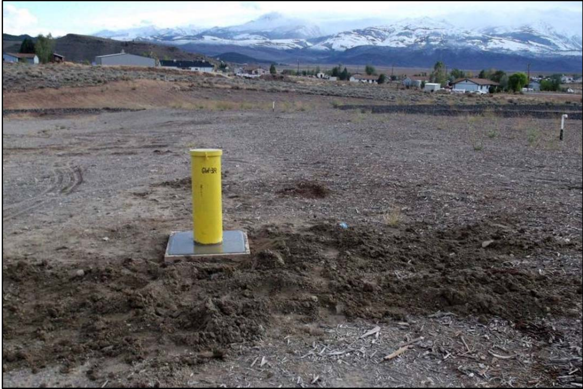
Plate 3-1. Landfill gas monitoring well GW-3R with LFG vent in final cover to right (view south).
