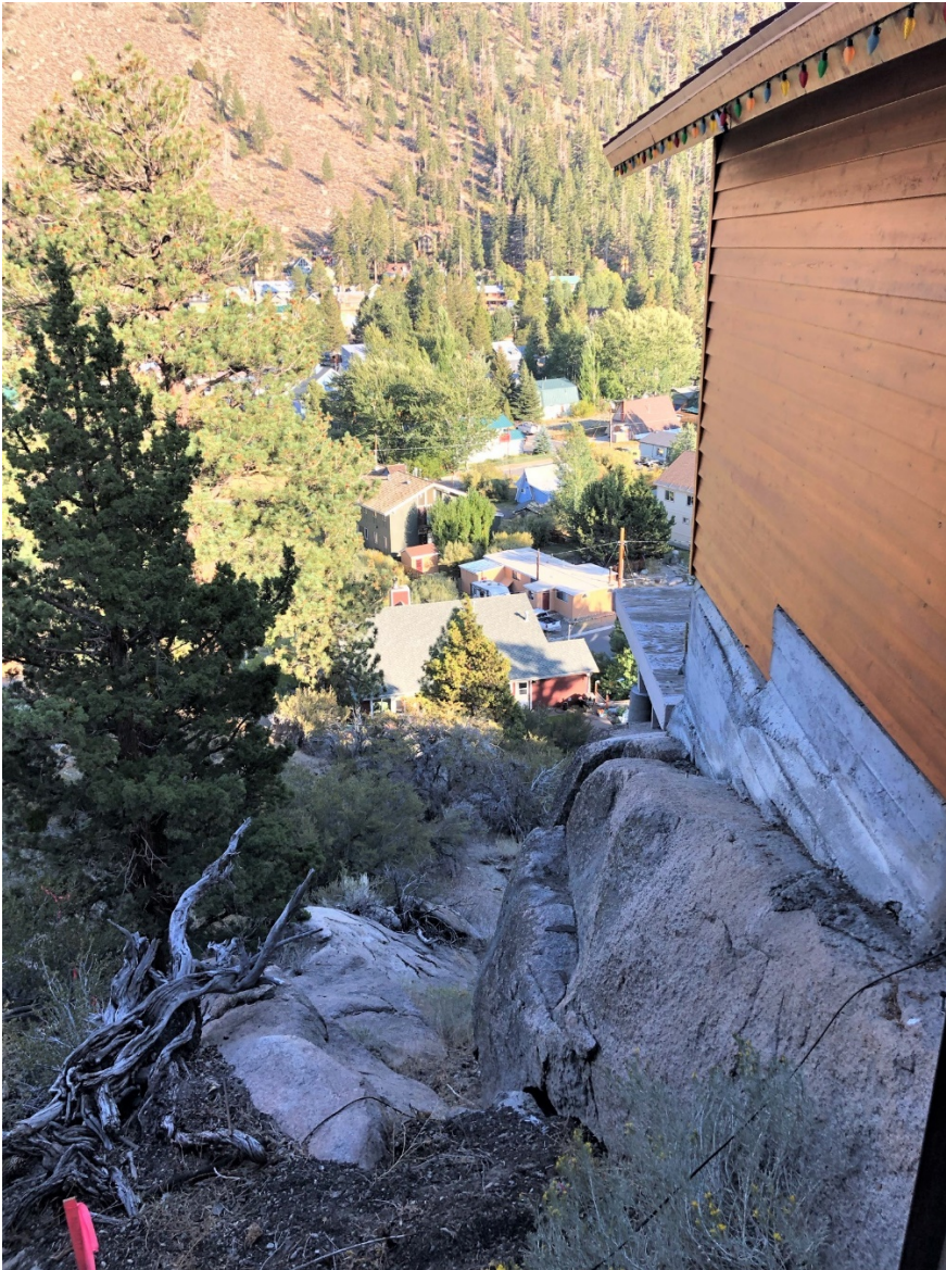
Figure 5. View along the north side of the house of the steep and rocky decline to the southeast
