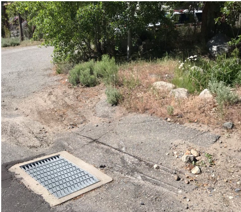
Possible emergency water draft point #2, a culvert located just outside of the project property line.
