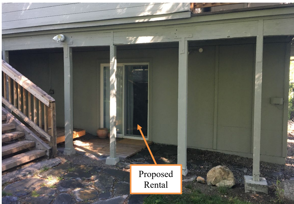
The proposed one-bedroom rental located on the ground floor at the base of the staircase.
