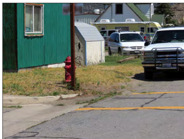
Sidewalks on School Street are missing or in poor repair.
