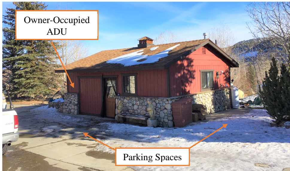
No exterior lighting observed on the owner-occupied ADU.
