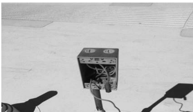
Electrical Image #14B – Junction Box without Cover
