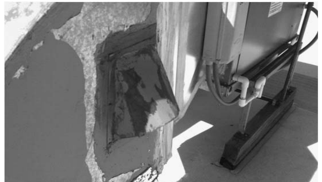
Mechanical Image 1 - Hooded outside air intake
