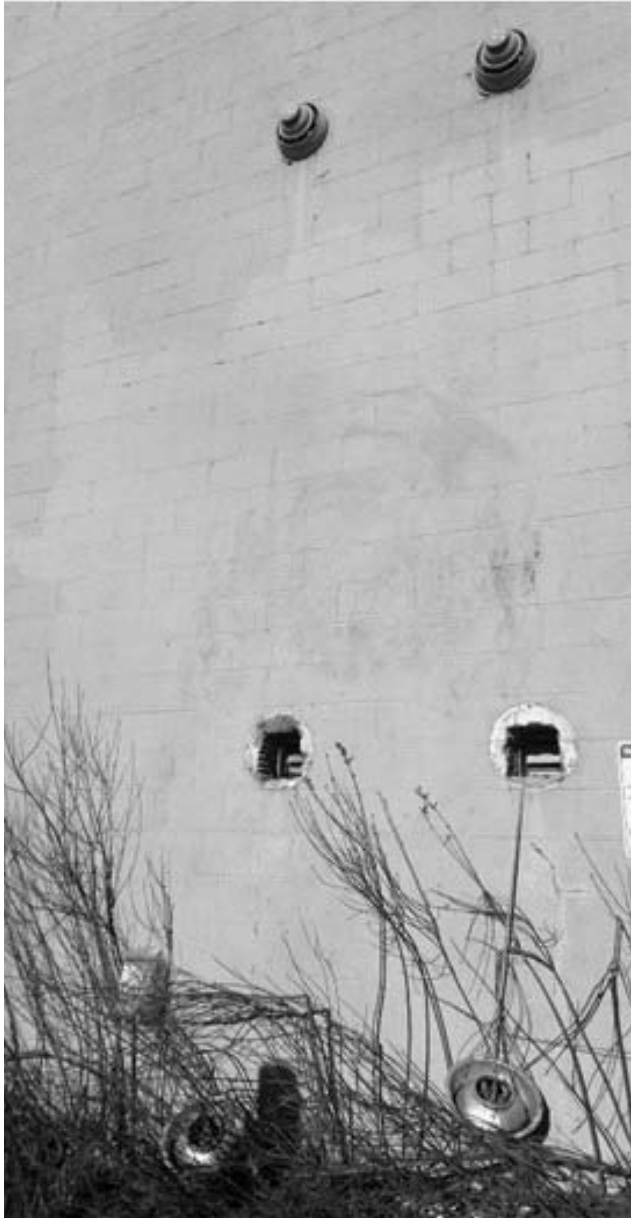
Mechanical Image 2 – Abandoned restroom exhaust fans
