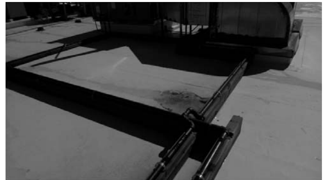
Plumbing Image 6 - Gas piping not secured to roof
