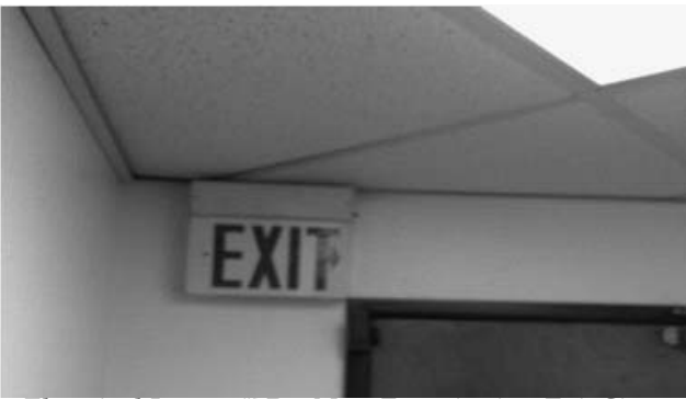
Electrical Image #7B – Non-Functioning Exit Sign
