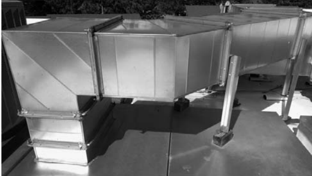
Mechanical Image 10 - No seismic bracing of ductwork and improper support
