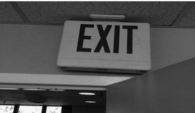
Electrical Image #7A – Non-Functioning Exit Sign
