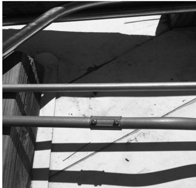
Electrical Image #15 – Set-Screw Type Fitting at Roof
