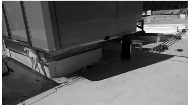
Mechanical Image 8 - RTU set on old curb and blocking without adapter and not properly secured to roof
