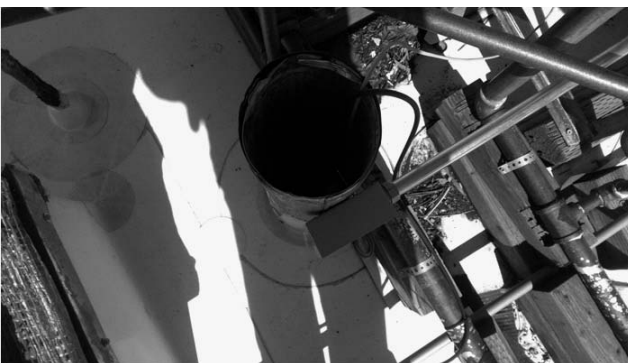
Mechanical Image 12 - Abandoned flue being used for electrical raceway
