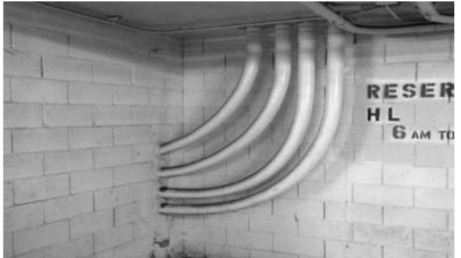
Electrical Image #2 – Southern California Edison Secondary Service Feeders at Parking Garage (Exposed)
