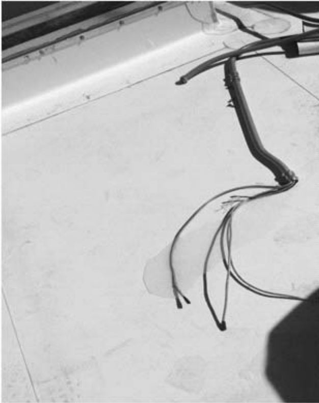
Electrical Image #13 – Exposed Roof-Top Branch Circuiting
