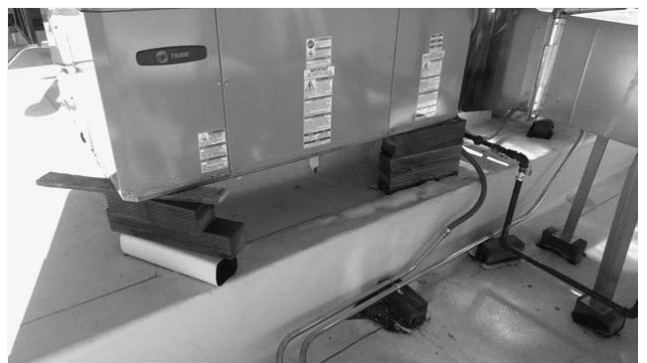
Mechanical Image 9 - RTU set on old curb and blocking without adapter and not properly secured to roof
