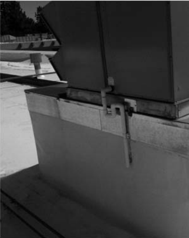
Plumbing Image 8 - Condensate to roof
