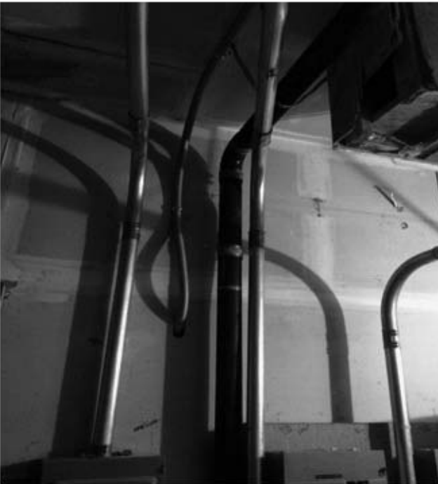
Electrical Image #4A – Sewer Pipe over Electrical Equipment
