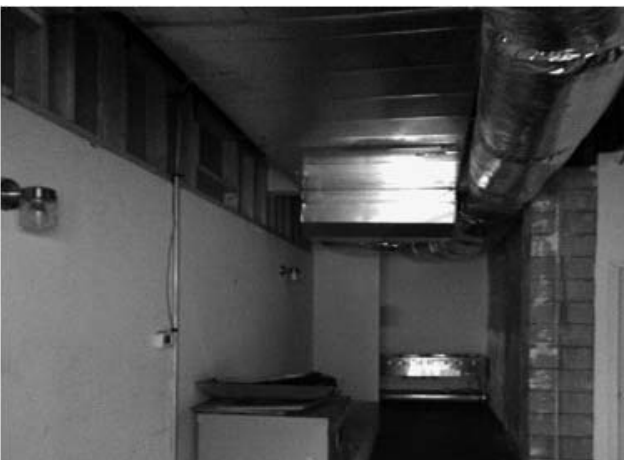
Electrical Image #4B – HVAC Ducting over Electrical Equipment
