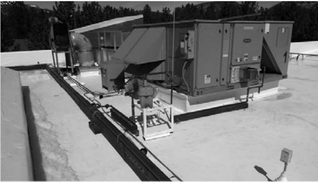
Mechanical Image 15 - Grease fan discharges toward outside air intake at RTU
