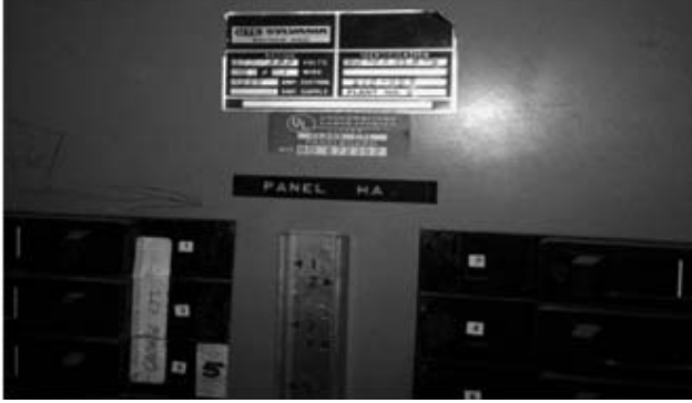
Electrical Image #3B - Missing Dead Front Cover
