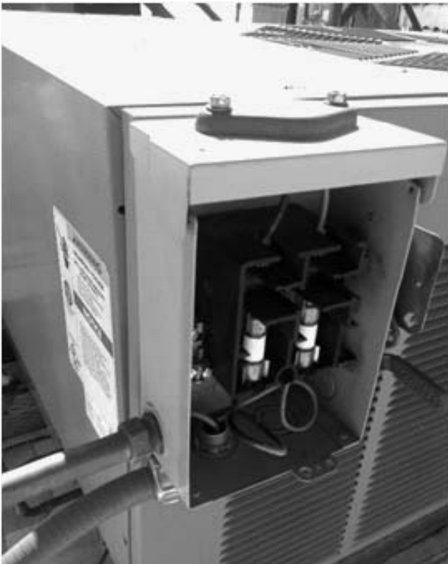
Mechanical Image 11 - No cover on fused disconnect switch
