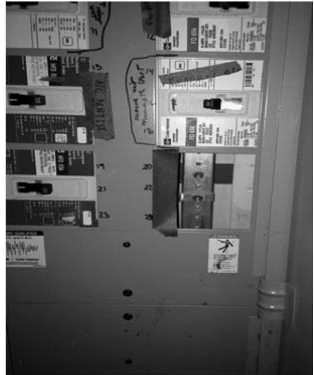
Electrical Image #3A – Exposed Live Bussing
