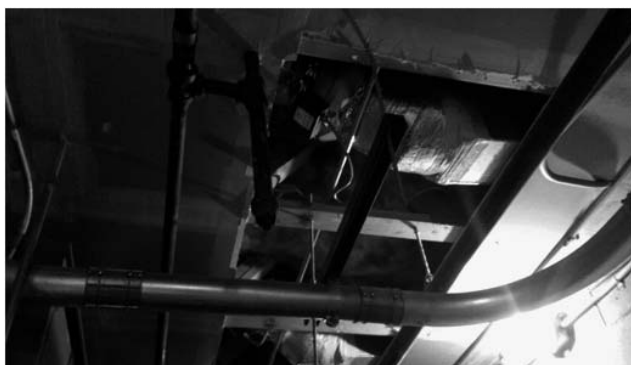
Mechanical Image 3 - Restroom exhaust fans
