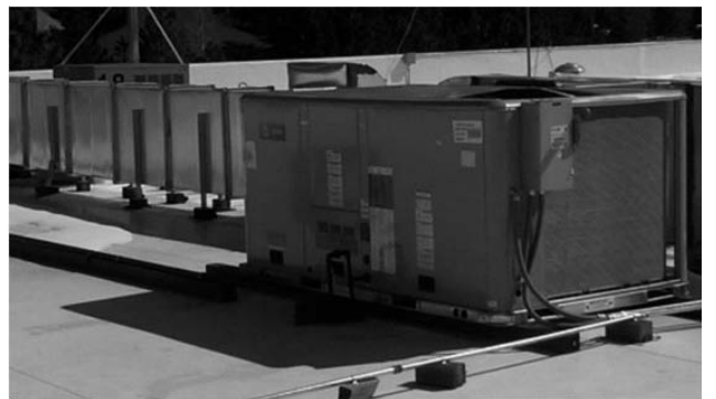
Mechanical Image 17 - No economizer installed on RTU
