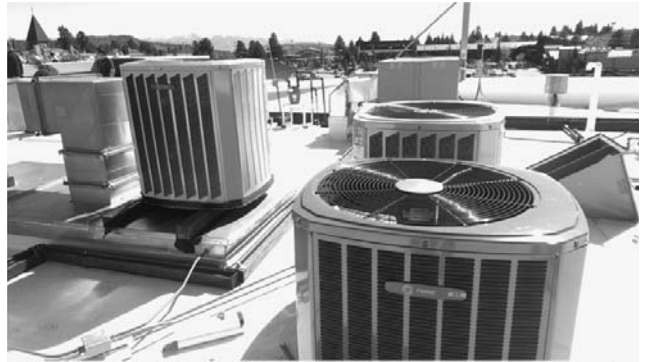
Mechanical Image 16 - Abandoned and unsecured condensing units
