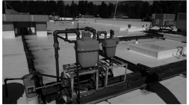
Plumbing Image 4 - Gas meters not supported
