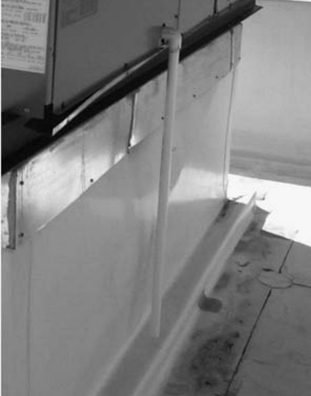
Plumbing Image 8 - Condensate to roof w/o p-trap
