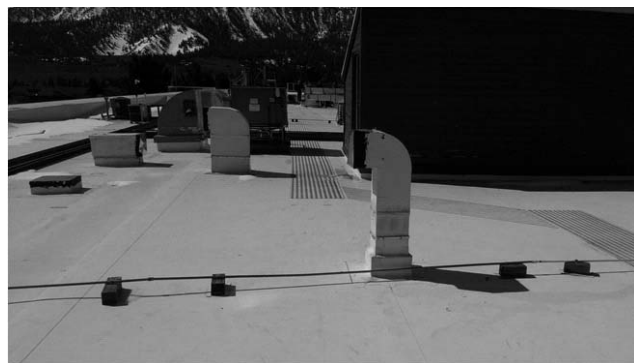
Mechanical Image 13 - Capped and abandoned ductwork on the roof
