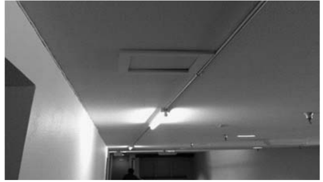
Electrical Image #8 – Surface Fluorescent Light Fixture and Raceway
