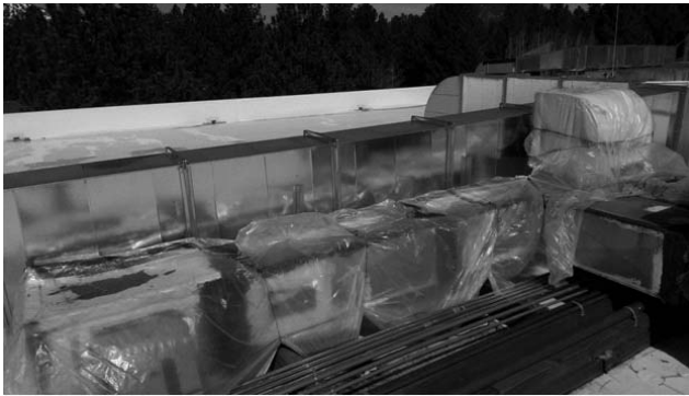
Mechanical Image 4 - Plastic wrap on ductwork
