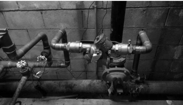
Plumbing Image 2 - Water main with backflow and saddle tap connection
