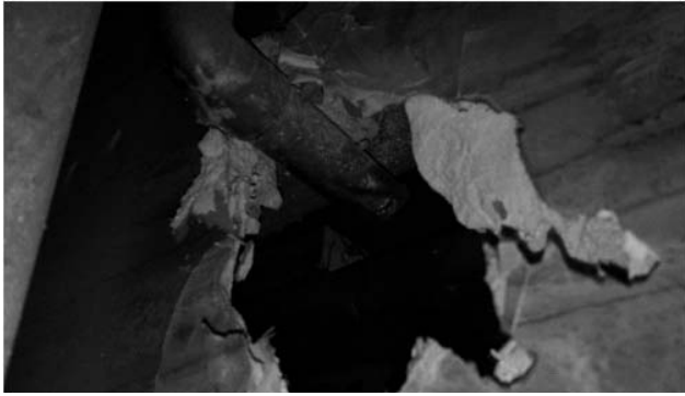
Plumbing Image 1 - Abandoned piping in the main electric room
