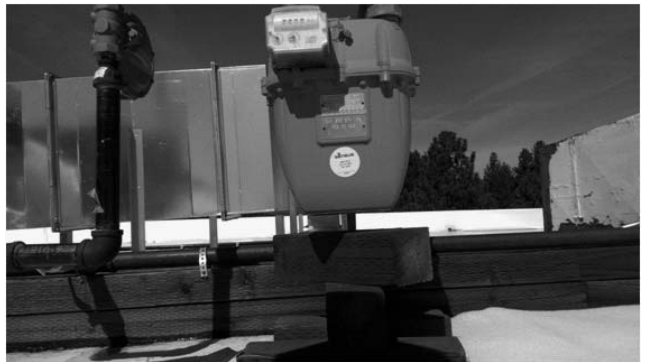
Plumbing Image 5- Gas meter not supported
