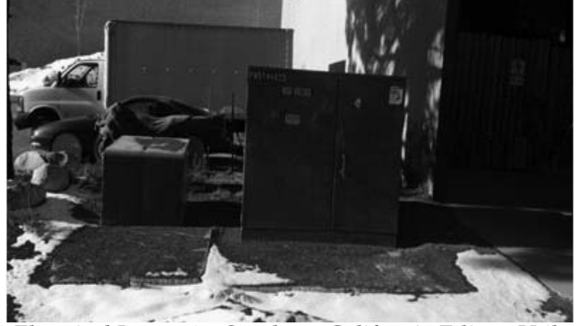
Electrical Image 1 – Southern California Edison Utility Transformer
