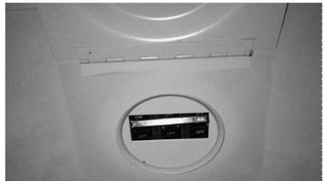
Electrical Image #5A – Proper Safety Switch
