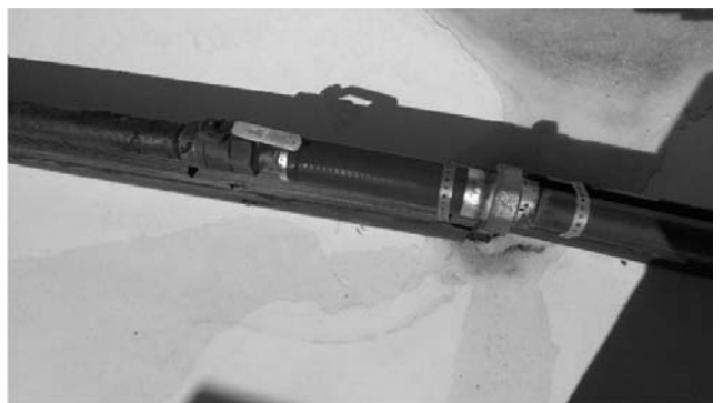
Plumbing Image 7 - Gas piping with non-approved tubing
