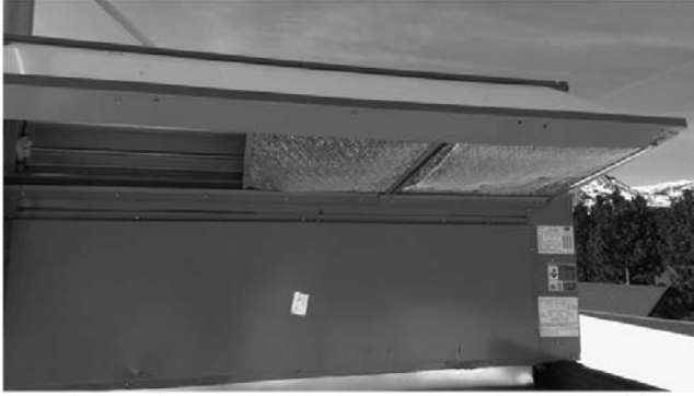
Mechanical Image 14 - Missing outside air pre-filter
