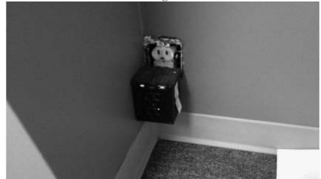
Electrical Image #10 – Duplex Receptacle with Missing Coverplate
