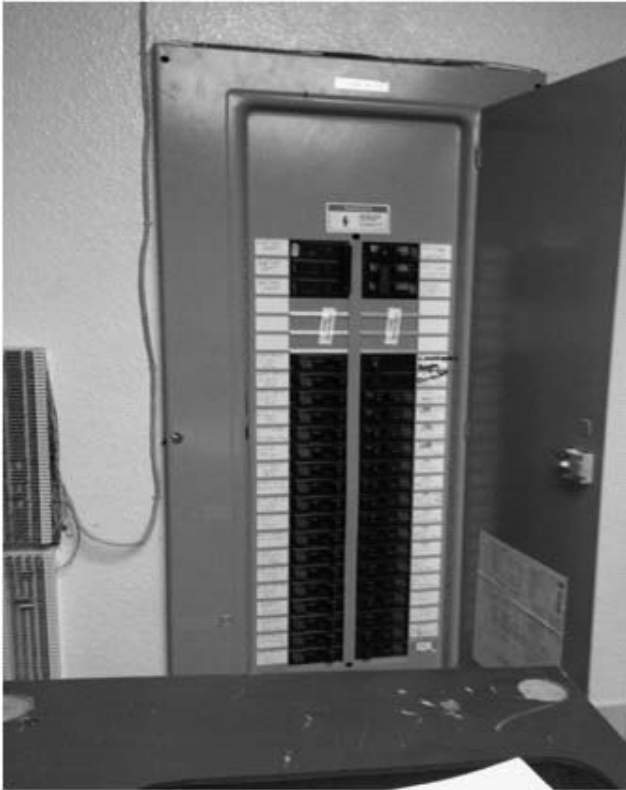
Electrical Image #6 – Improper Panelboard Mounting
