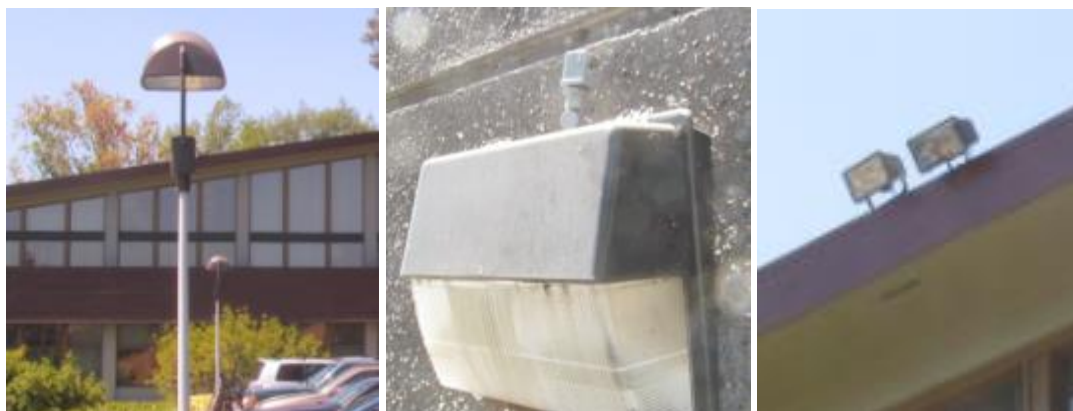
Figure 3.5: Metal Halides Fixtures (left) and High Pressure Sodium (middle and right)
