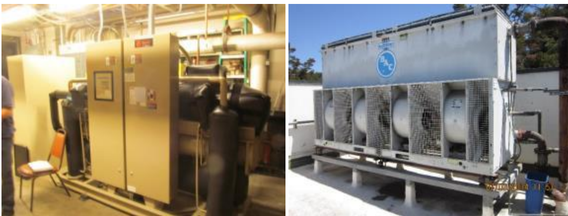
Figure 3.3: Trane Screw Chiller (left) and BAC Cooling Tower (right)
