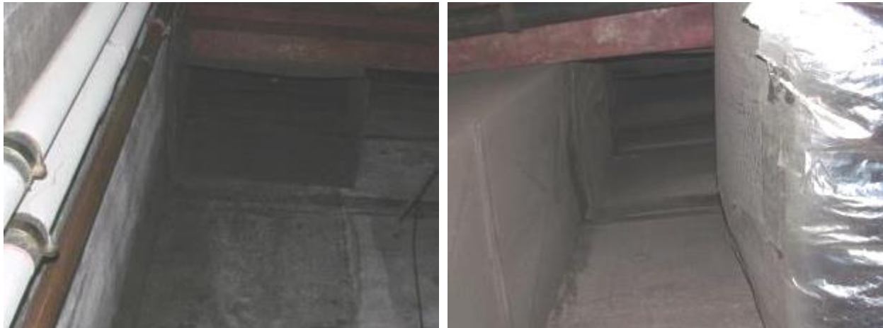
Figure 5.1: Outside Air Inlets for AHU-1 (left) and AHU-2 (right)
