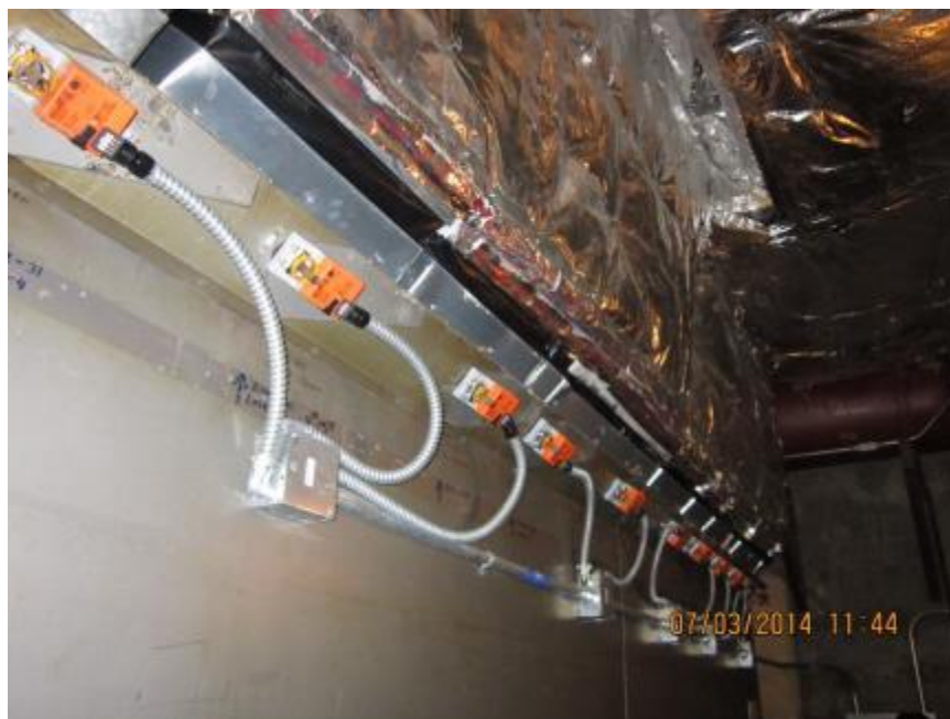
Figure 3.2: AHU-2 Zone Mixing Dampers on the Air Handler Discharge
