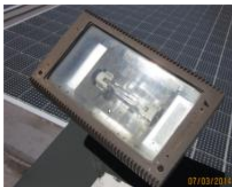
Figure 5.7: High Pressure Sodium Flag Light
