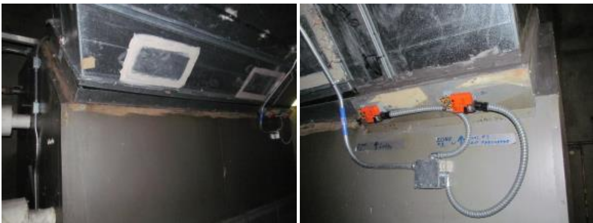
Figure 3.1: AHU-1 Hot and Cold Decks (left) and Zone Mixing Dampers (right)
